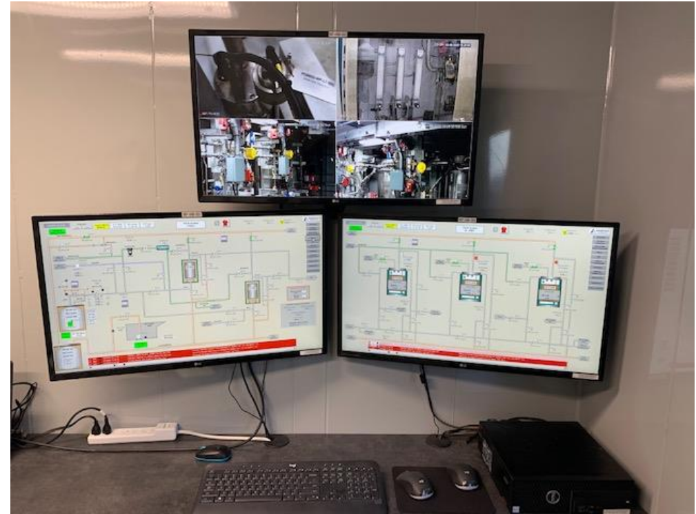
TSCR HMI-Control Station
