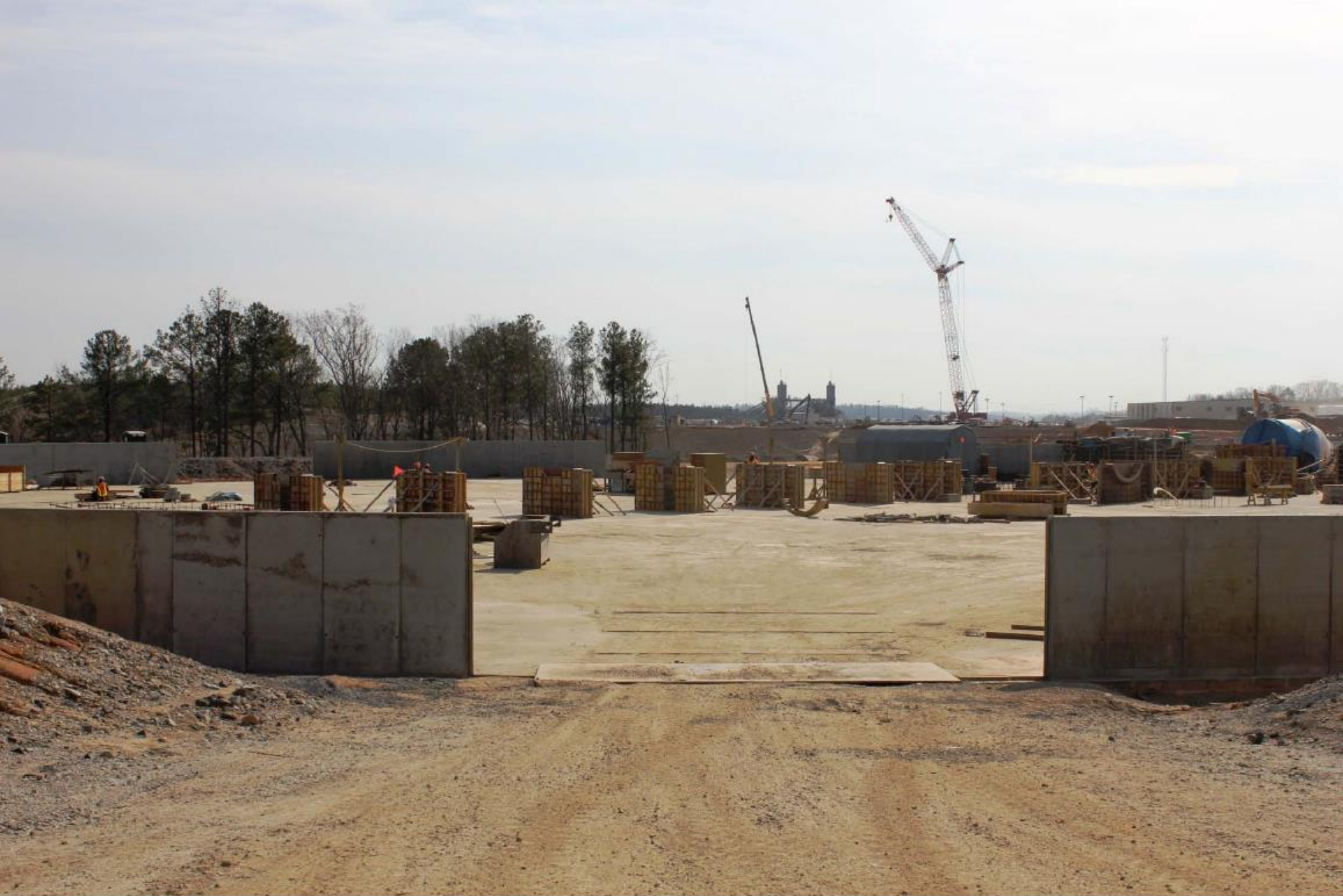
02. 09.12 Cooling Tower 2A
